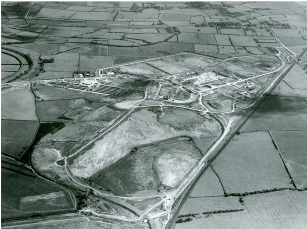
Plate 17: View of West Burton Power Station taken in 1961 during construction, facing south
