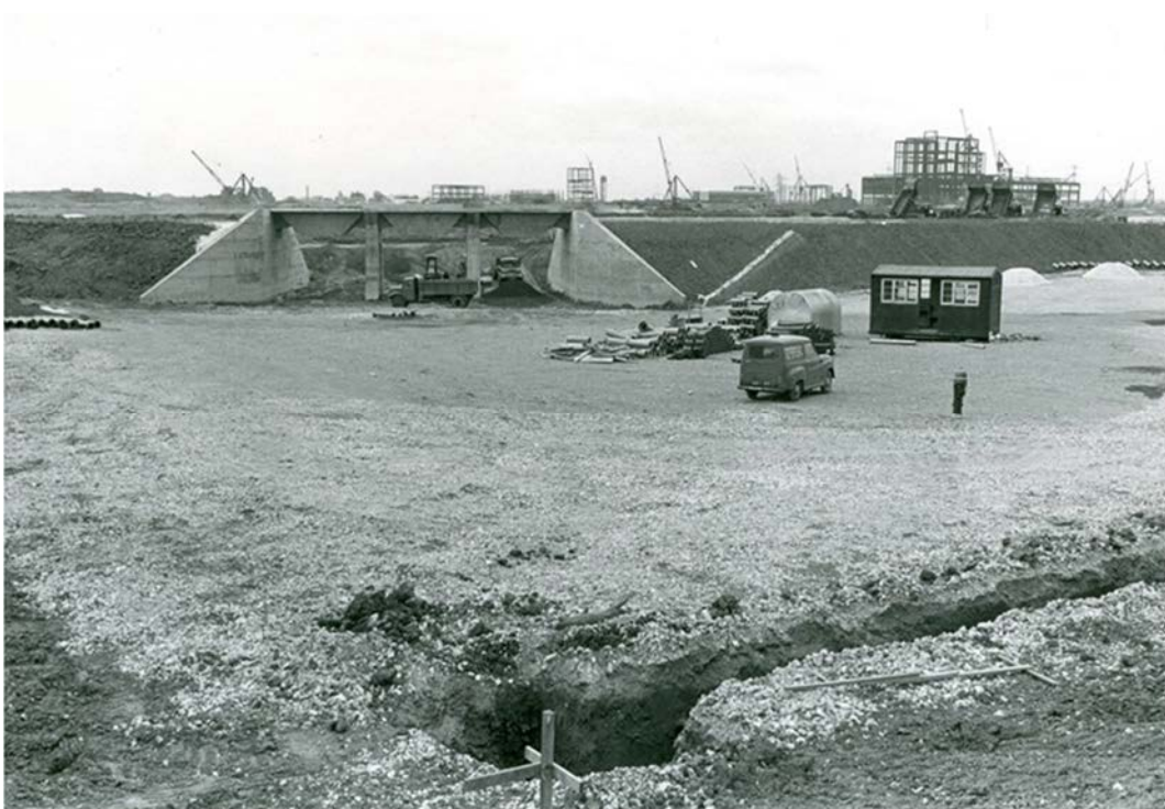
Plate 19: The Emergency Coal Discharge Bay immediately north of the Coal Storage Area, facing south-east
